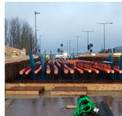
In Brøndby, work began on the construction of a new bridge across the Copenhagen-Ringsted track.
