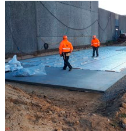
In 2018, the work began to establish a pedestrian tunnel below the suburban-train line at Buddinge Station.
